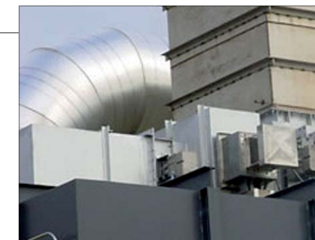
Secondary heat recovery system returns energy to process or other plant energy requirements
