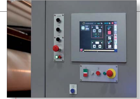
Control panel and WEBVIEW.
