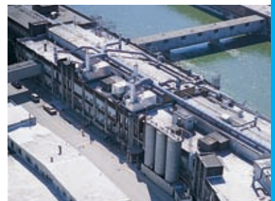
The lightweight MEGTEC MAGNUM offers flexible installation. Roof-mounting saved this plant considerable cost in ductwork.
